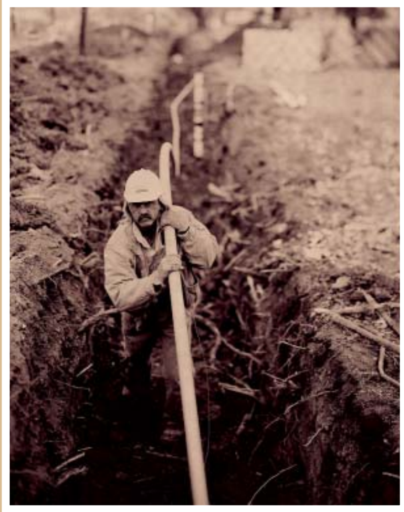
RAY WETZBARGER IS AN XCEL ENERGY SERVICE FITTER APPRENTICE IN GRAND JUNCTION, COLO.
